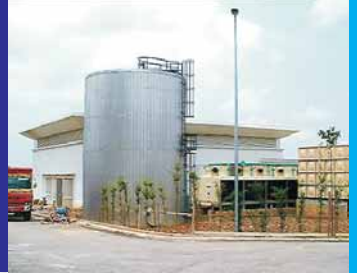
University Telekom, Melaka Capacity: 5,800RTh, Size: 23' Dia x 32' H
